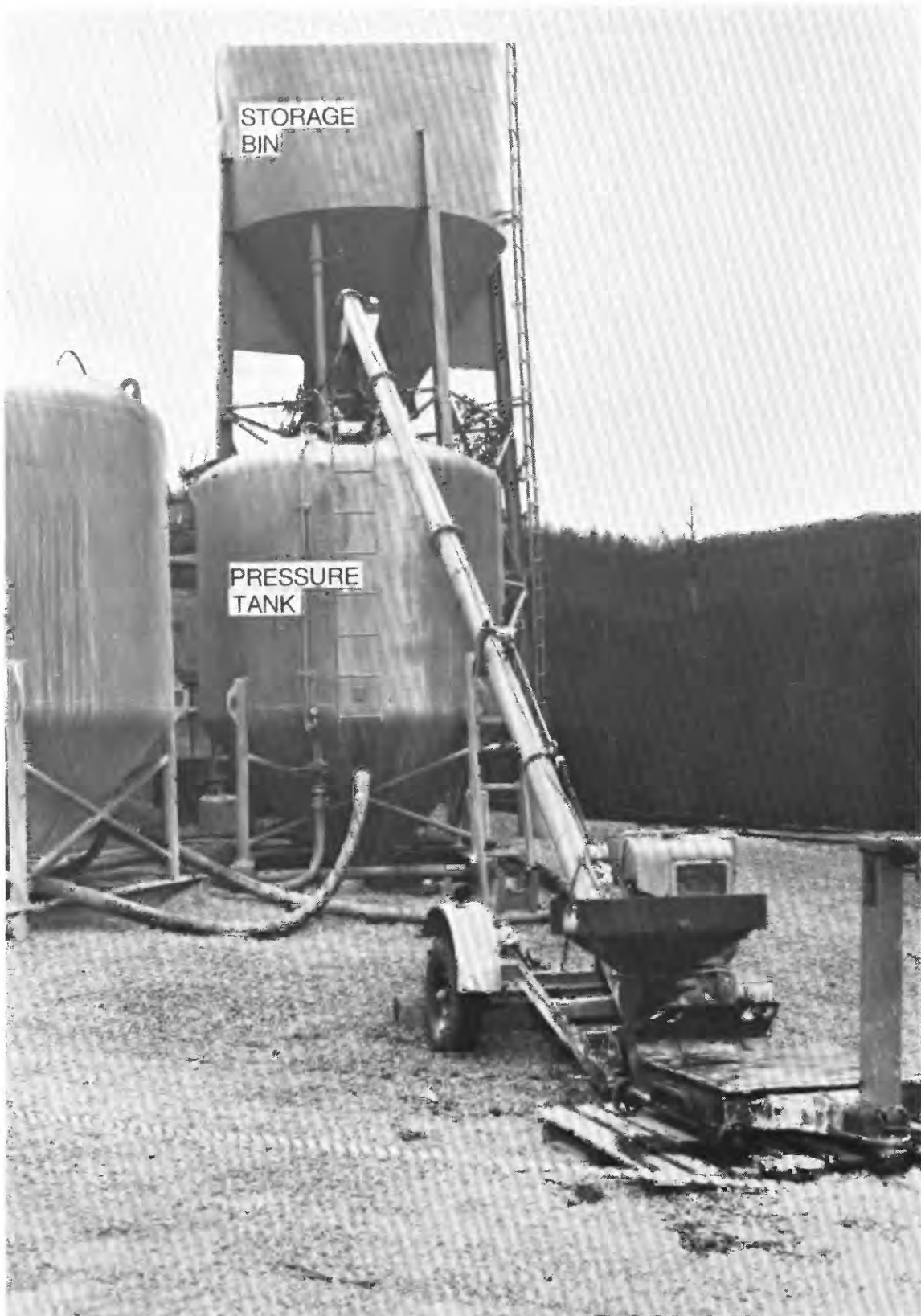
FIGURE 41.—Photograph showing equipment for proportioning and blending dry solids for waste-grout injection, Oak Ridge National Laboratory, Tenn. (Courtesy of Oak Ridge National Laboratory.)
