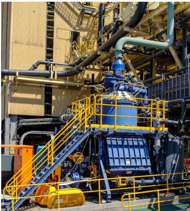
Figure 3. RFC2000 installed on-site
