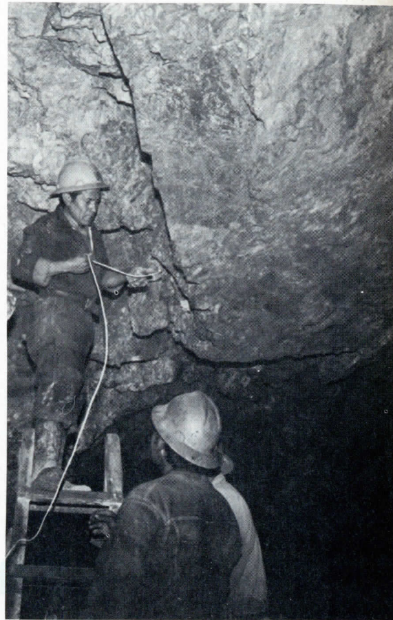
CHARGING up blastholes at the Madrigal mine, where Santa Rosa is main vein.
