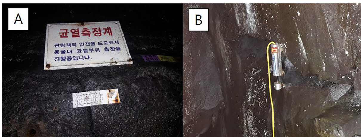
Fig. 2. Crack monitoring using glass plate (A) and monitoring gauge (B) in Manjanggul Cave (lava tube), Jeju Island, Korea.
