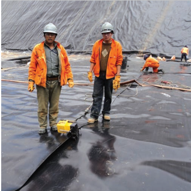
El Aliso workers installing liner materials at Yanacocha. (Photo courtesy of El Aliso)
