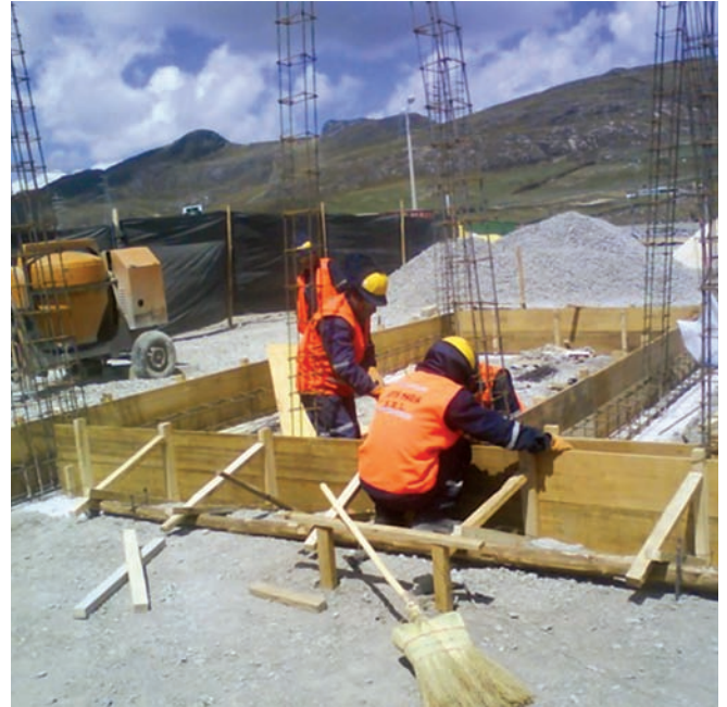
Santa Maria Hualgayoc workers at a construction project at Cerro Corona. (Photo courtesy of Santa Maria Hualgayoc)
