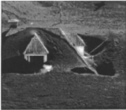
House on Heimaey buried by ashfall, but roof is still intact due to strong design and steep slope.
